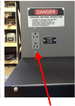
120VAC receptacle for pump
