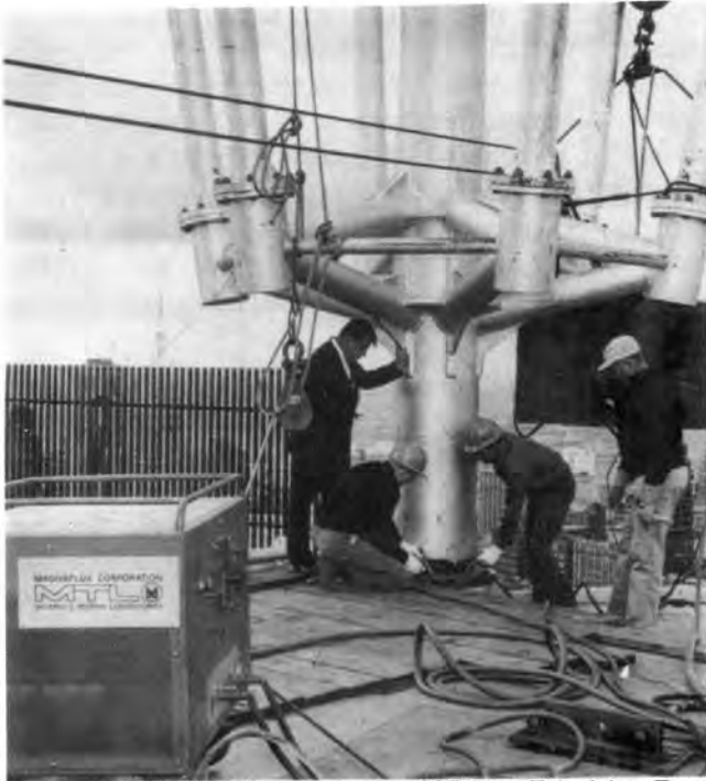
Fig. 222—Testing Weld at the Base of a 285-Foot Television Tower on the Roof of One of the Twin Towers of Marina City in Chicago.
