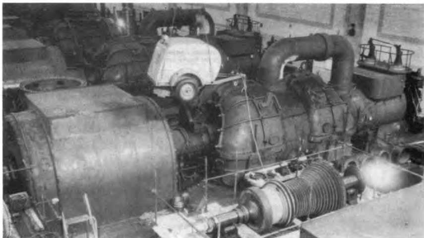
Fig. 208—Preparations for Testing Steam Turbine Spindle and Blading for Cracks.
