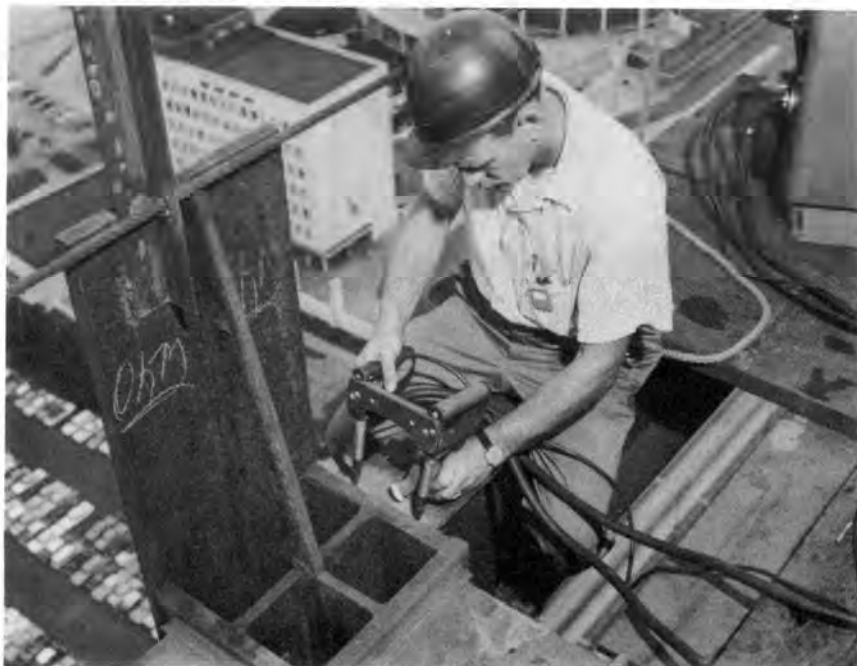
Fig. 221—Inspecting Welds with Magnetic Particles on the 32-Story Michigan Consolidated Gas Company Building in Detroit, Michigan.
